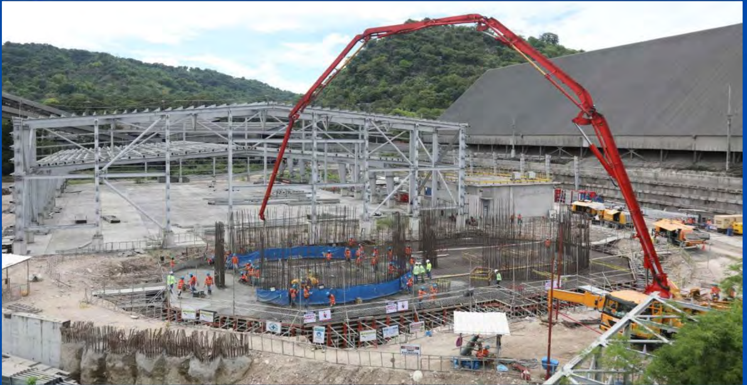
Concrete foundation pouring for cement silos in Solid Plant New Line project Built with Rizal Vertua® Classic High Strength cement
