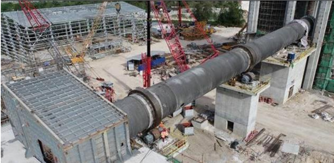
New rotary kiln at Solid Cement Plant
